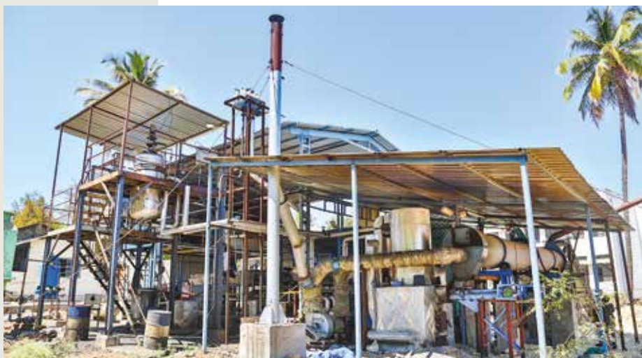
TCTD plant situated at TKIET, Warnanagar
